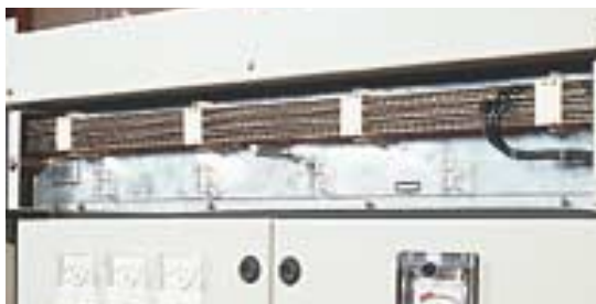
Auxiliary busbars in front of main busbar compartment.
