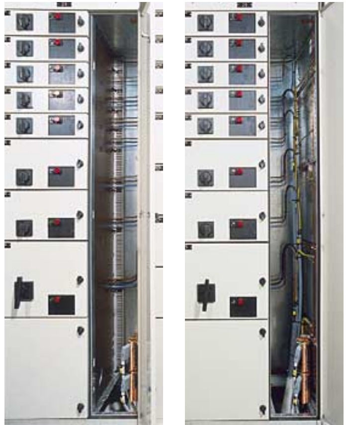
Cable-entry compartment left: cable entry through screening plates; right: cables supported by strip-mounted cable clamps.
