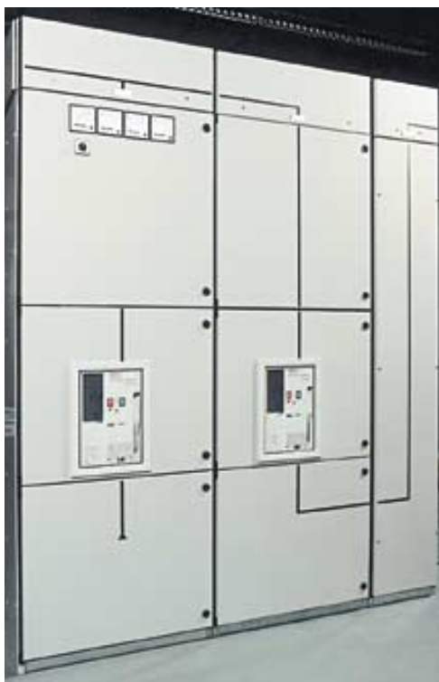
Capitole 40 assembly with Aeromat air circuit breakers as incoming feeder and buscoupler.
