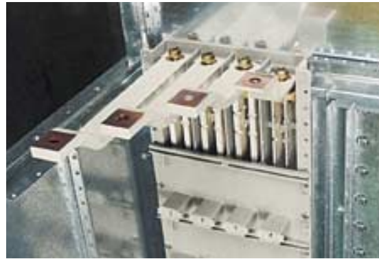
Distribution busbar duct with connection bars to main busbar system (upper sealing plate removed).
