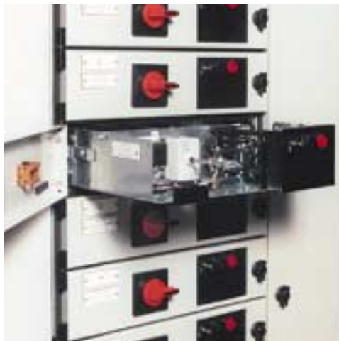
Capitole 40 cubicle showing partly withdrawn motor starter tray.
