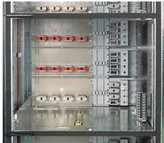
Switchgear and controlgear compartments for drawout units, showing from left to right: scissor contacts to distribution busbars, sockets to auxiliary busbars, and cable terminal blocks.
