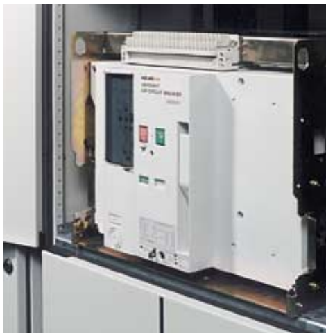
Close-up view of Aeromat air circuit breaker in Capitole 40 cubicle.
