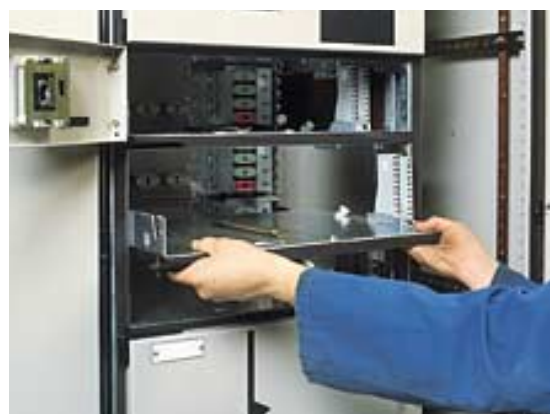
Changing of outgoing compartment sizes can be safely carried out under live conditions.
